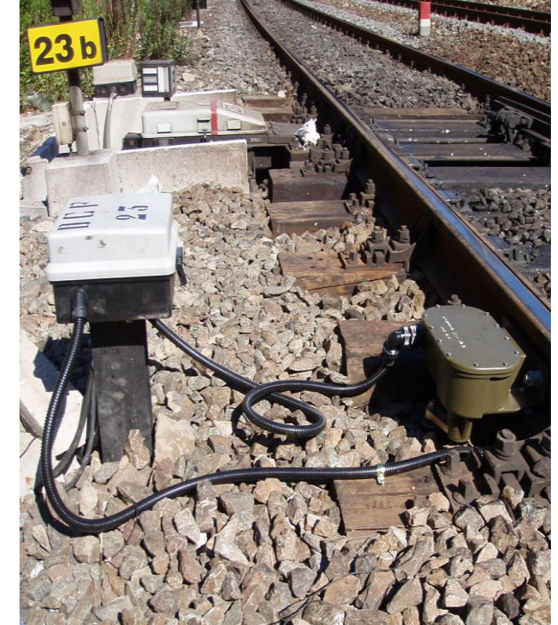
Italy (Point control box)
