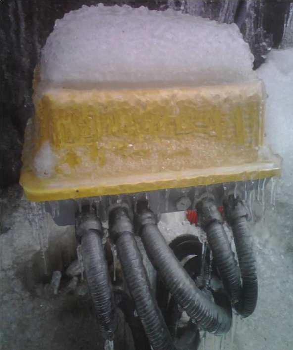
Spain (Signal junction box)
